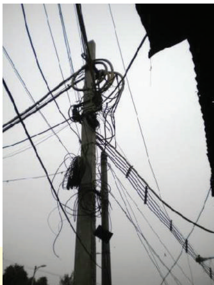
Street light clustered with wires without lamp post (Ajmeri Gate site)
