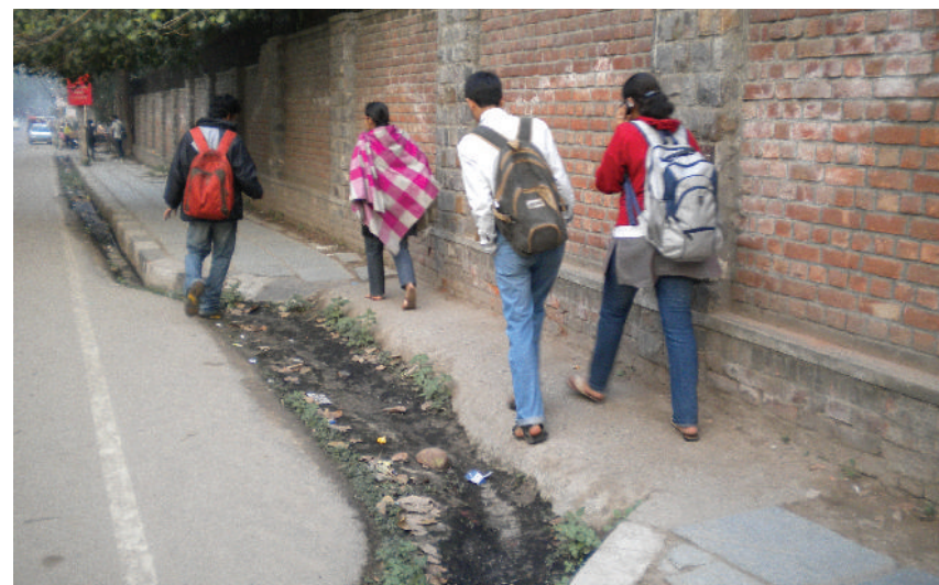
Broken/ Narrow Pavements in New Delhi
