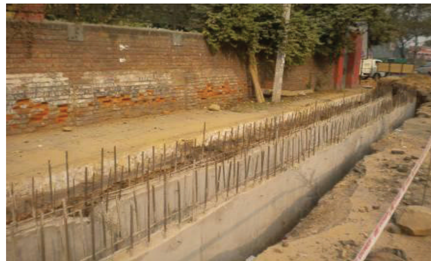
Under construction site along the busy lane towards Kamla Nagar Market in University of Delhi (North Campus)
