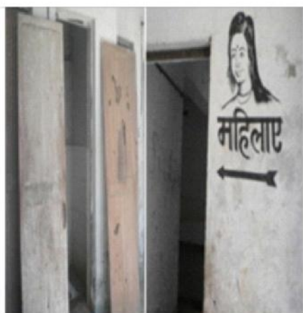
Broken doors of women's toilets
